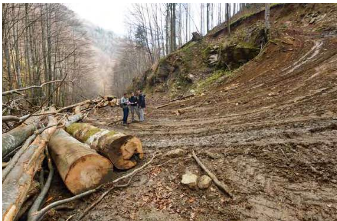
Bulldozing of logging road through the buffer zone of a UNESCO World Heritage site within Domogled - Valea Cernei National Park.
