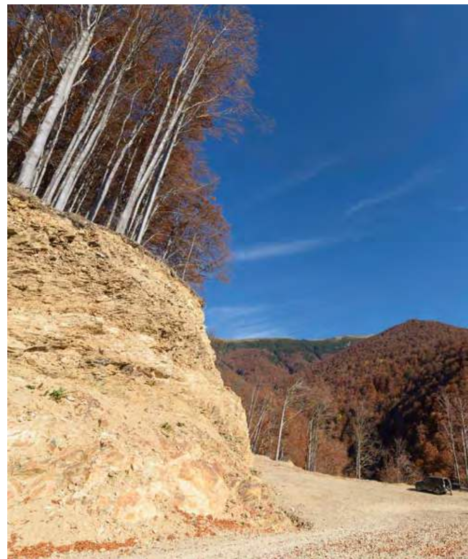
EU funded road construction in a pristine valley in the Vâlcan Mountains, Nordul Gorjului de Vest Natura 2000 site.
